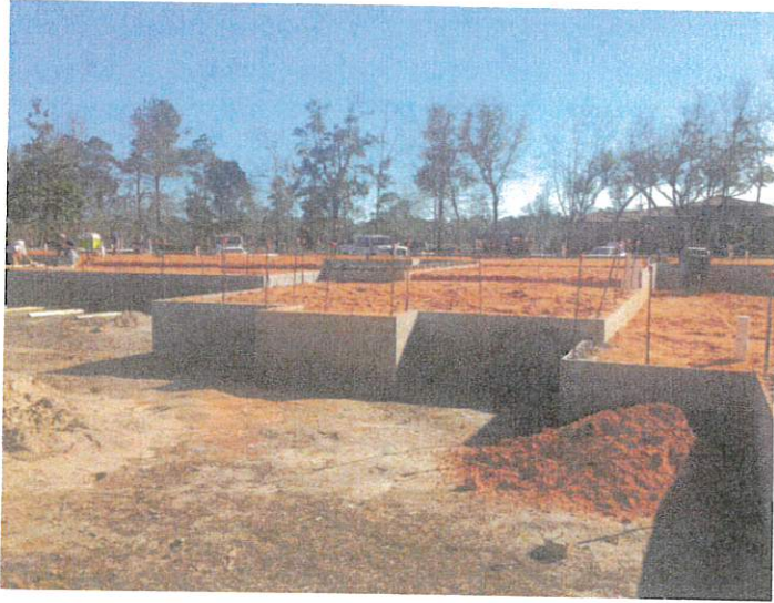
Rear view of Hyde residence under construction 1/29/15, looking South, Lots 51 & 52, Waterside Subd., City of Gulfport, MS.
